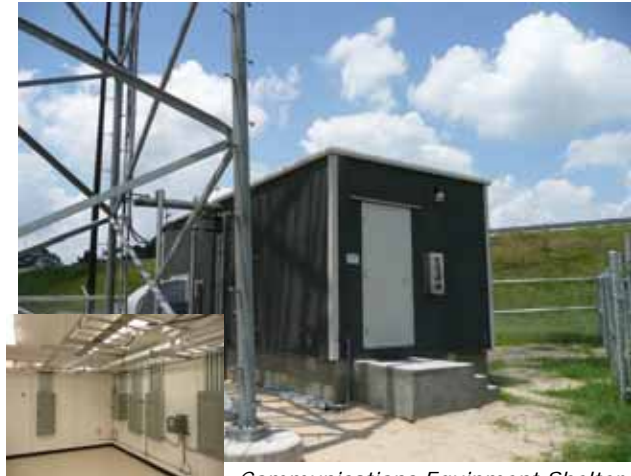
Communications Equipment Shelter
